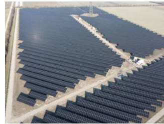
EVN Trumau 9.996 kWp
